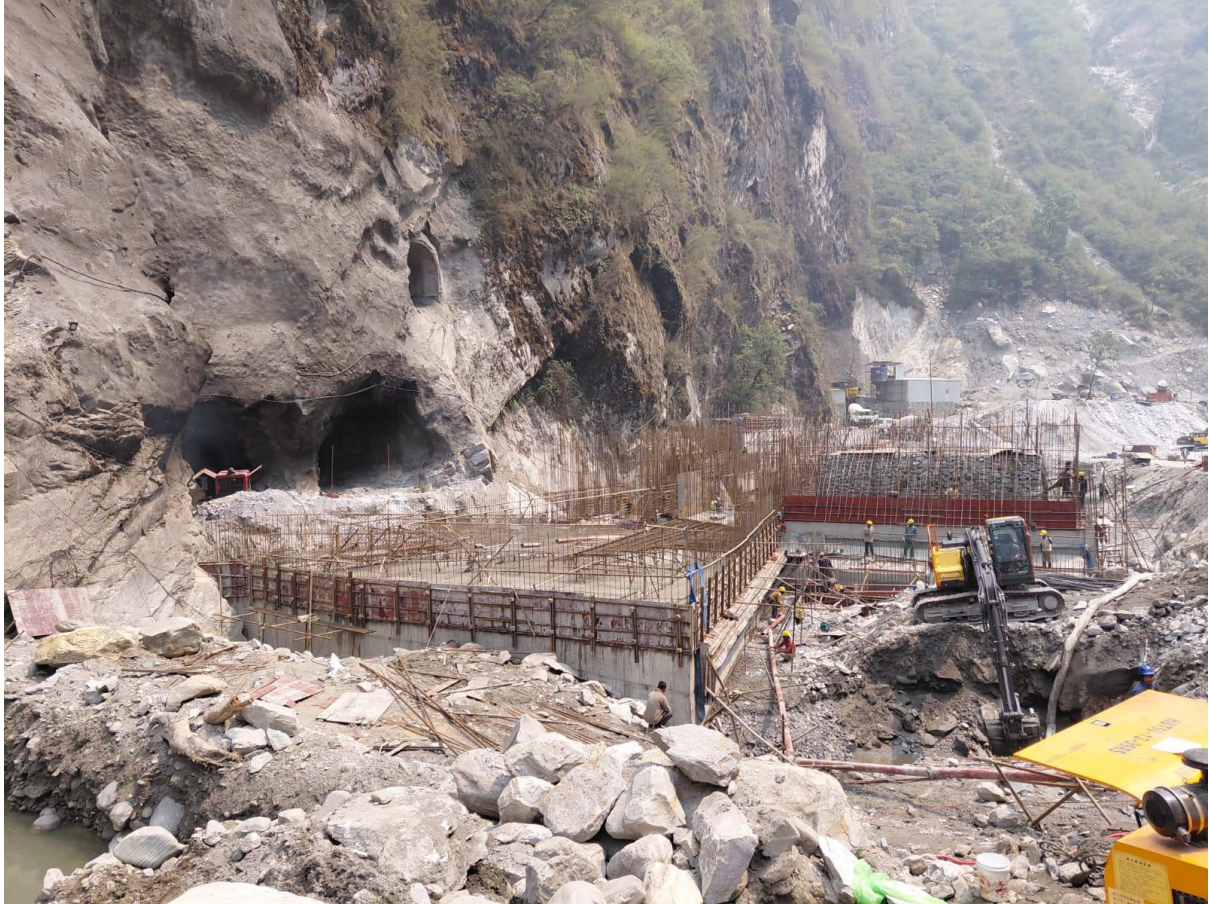
Figure 3: Intake Orrifice gate raft
